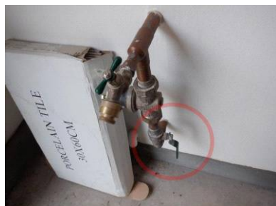
The main water shut off valve
