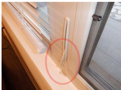
Damaged latch handle
