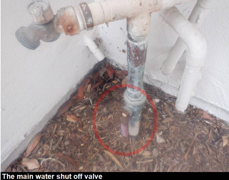
The main water shut off valve
