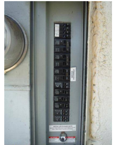
Label the breakers
